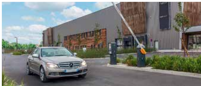
AUTOMATIC STREET BARRIERS
